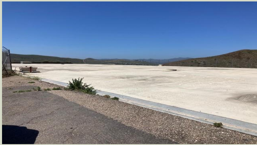
Lindero Reservoir (4 MG)
