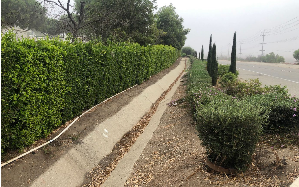
Photograph 7. Unnamed Feature No. 9. Concrete roadside ditch along Tierra Rejada Road. View facing northeast. October 6, 2022.
