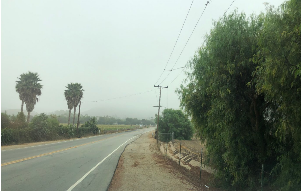
Photograph 3. Unnamed Feature No. 8. Concrete-lined roadside ditch along Sunset Valley Road. View facing southwest. October 6, 2022.
